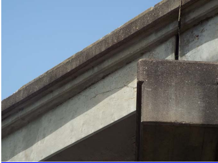
BEAM A - SPAN 2 - CRACK
