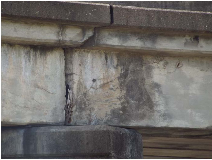
BEAM K - CRACKS AT BENT 1
