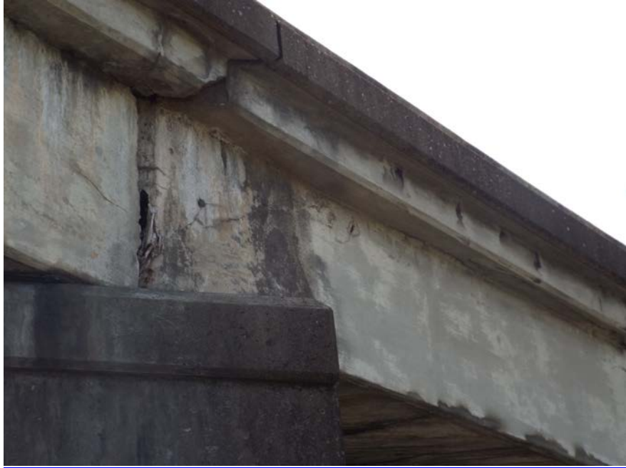
BEAM K - CRACKS AT BENT 1
